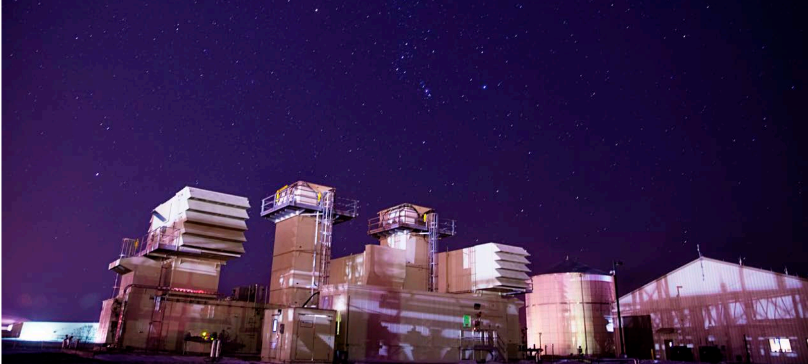
The Aberdeen Peaking Plant helps us respond to changing load conditions.
